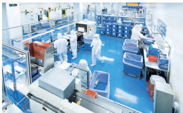
Injection molding and assembly of inhaler in the ISO 14644-1 ISO class 8 clean room in Dongguan City, China
