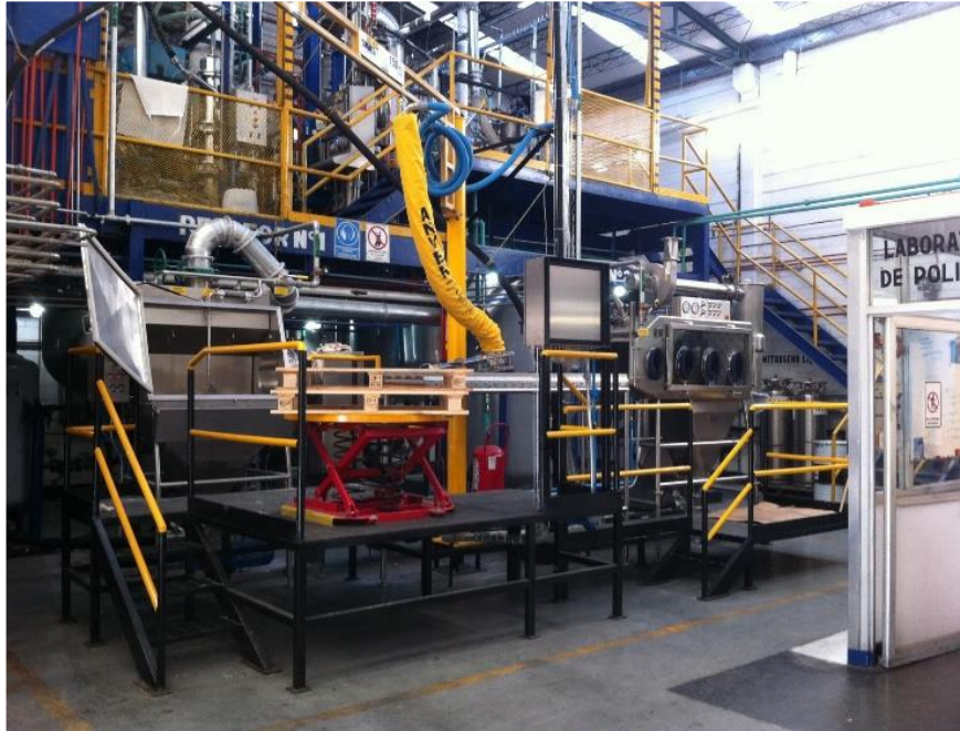
Sack cabinet and Isocharge for bag discharge
