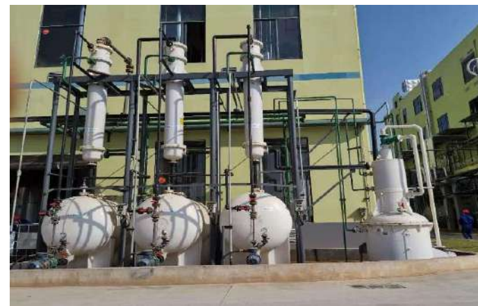
Acid Waste Gas Treatment - Falling Film Absorption + Alkali Absorption
