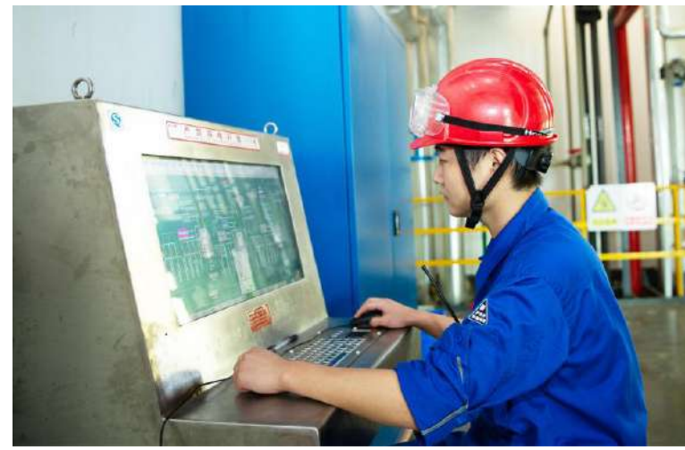
DCS & SIS control console
