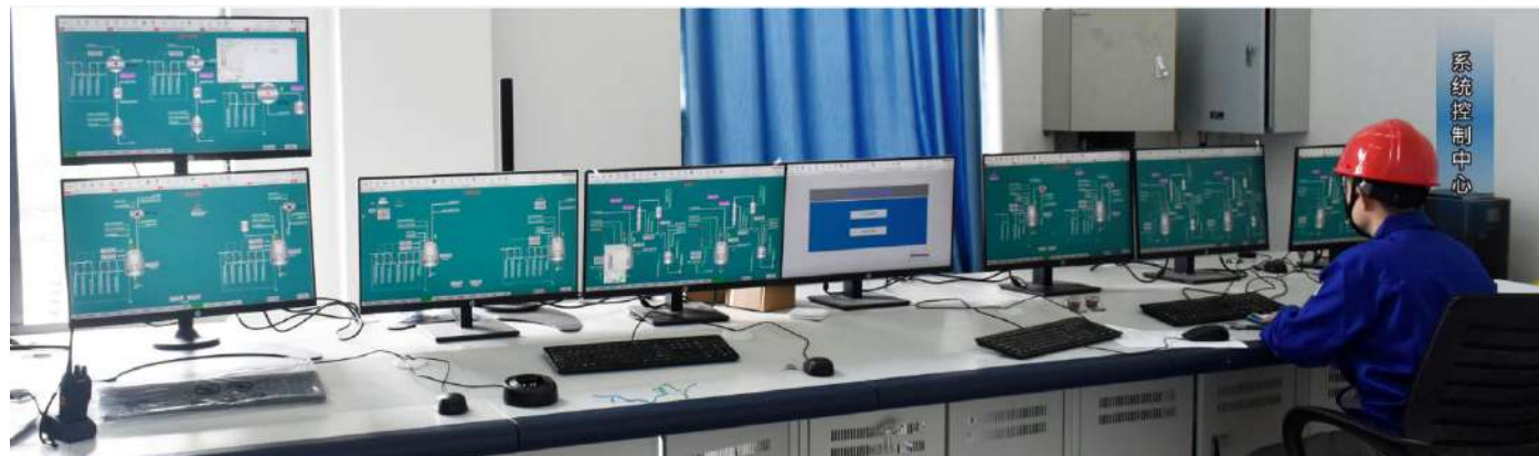
System control center
