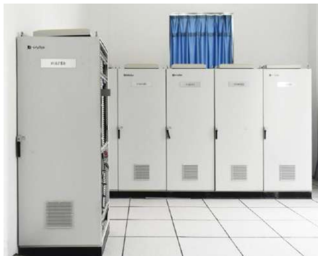
DCS & SIS system equipment room
