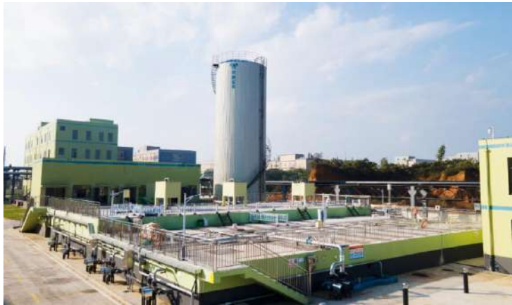
Wastewater Treatment - TIC Anaerobic Reactor
