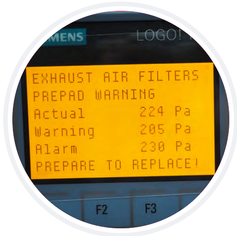
Integrated PLC Control System
