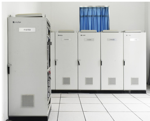
DCS & SIS system equipment room
