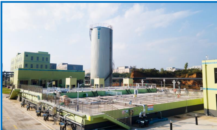
Wastewater Treatment - TIC Anaerobic Reactor
