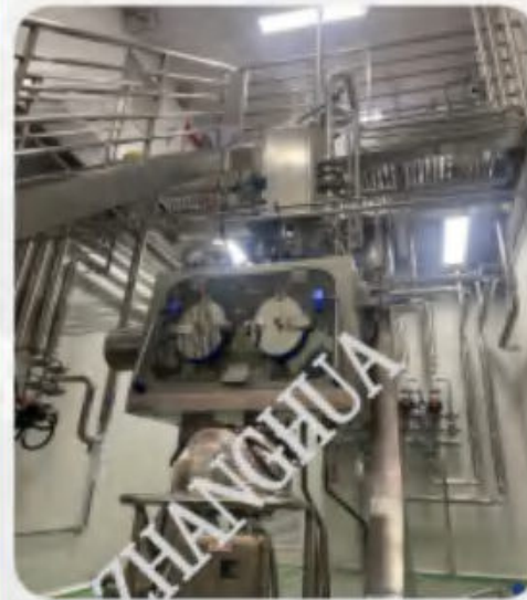
ANFD with special isolator
