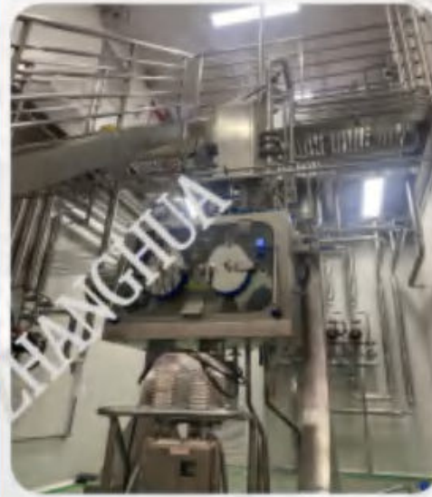
ANFD with special isolator
