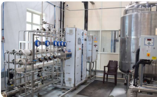
WATER PURIFICATION SYSTEM
